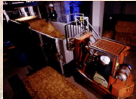
The hammermill: Area where straw is mulched into a powder, increasing the surface area, which allows the cellulose to be easily attacked by enzymes.
