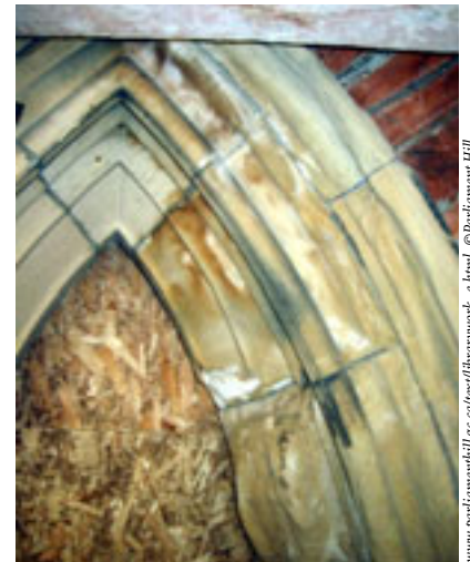
Example of damage (efflorescence – seen as a powdery deposit) on the stone arches.
